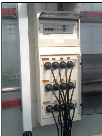
Figure 2. The main switch of the automated system.
